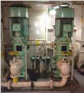
Lubricant oil, 150m 3 /h, 4bar Pump installed inside the vessel.
