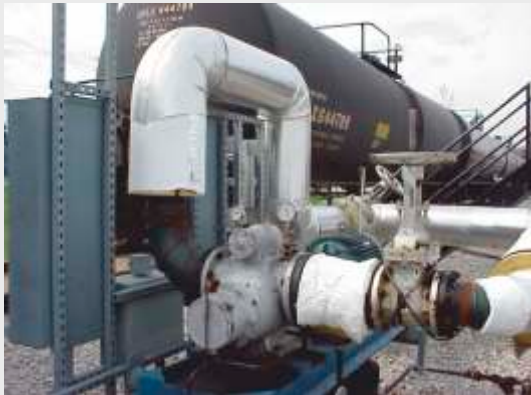
Multi screw pump for Refinery Asphalt, 120m 3 /h, 10 bar Heating system
